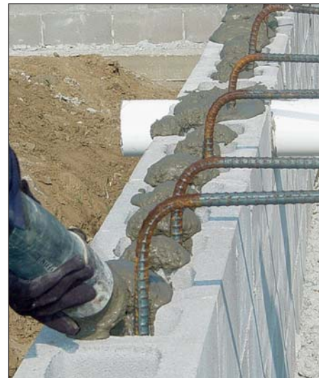
FIGURE 4. In termite-infested locations, every core in any block wall should be fully grouted.
