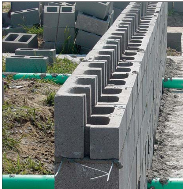
FIGURE 3. Lacking locally available L-blocks, a builder in Louisiana resorted to cutting standard-size blocks to create the slab form. While effective, this work-around increased the cost of completion.
